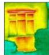
Poorly fitting windows and "thermal bridging"
